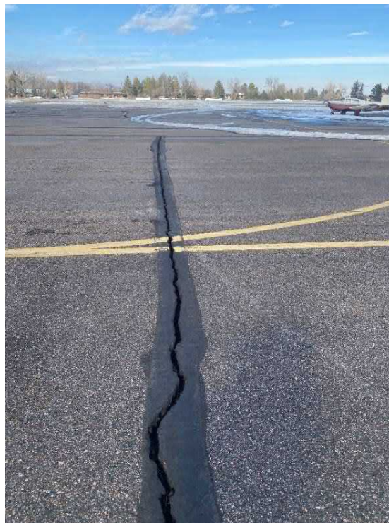
Figure 4. East Terminal Apron Longitudinal Cracking
