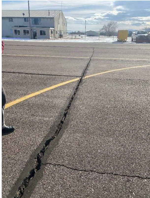
Figure 2. Central Terminal Apron Longitudinal Cracking
