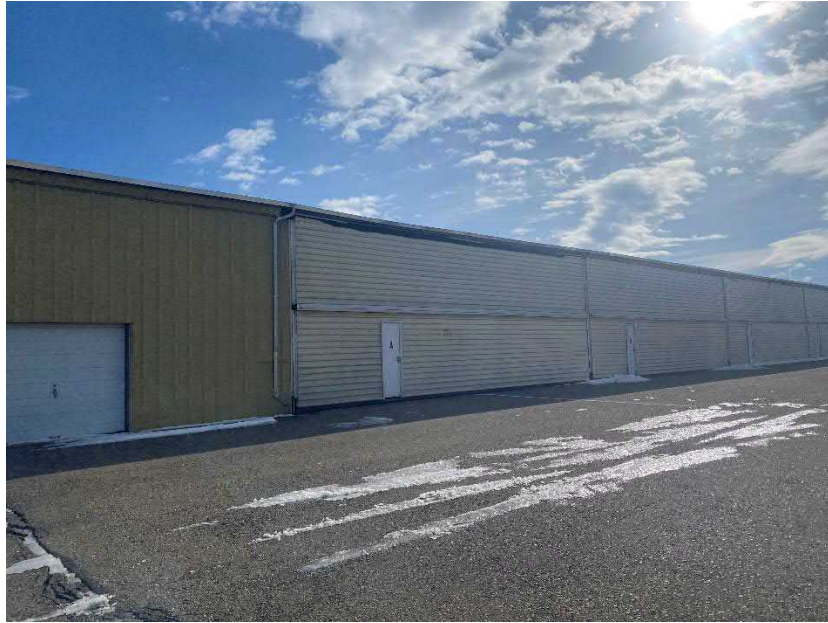
Figure 9. East T-Hangar Exterior, Door, and Gutter Conditions
