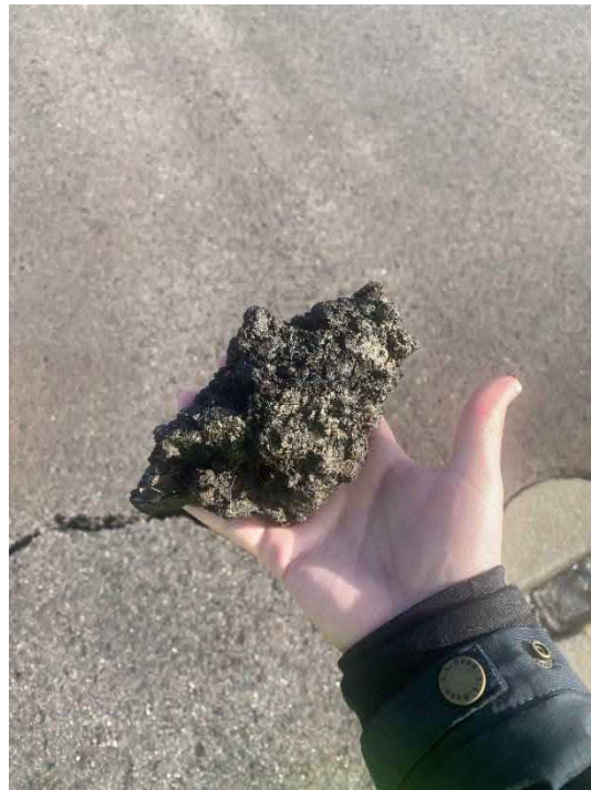
Figure 5. East Terminal Apron Foreign Object Debris (FOD)
