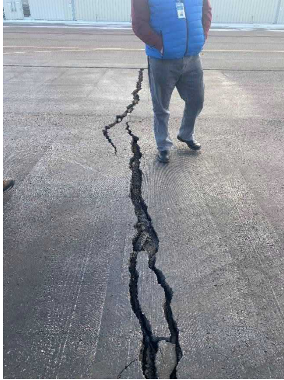
Figure 3. Central Terminal Apron Major Longitudinal Cracking
